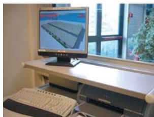
Introduction of a heating control system
