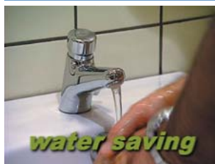
Saving water with a new automatic faucet
